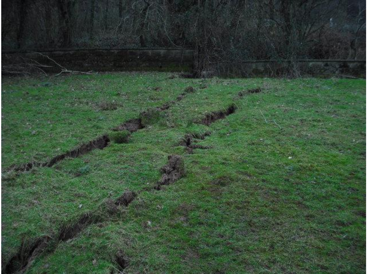
View of retaining wall showing extent of ground movement
